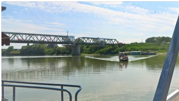
Figure 2 The works on the Po Bridge and the small new ferry, for the small passage (Photo Galvani).
