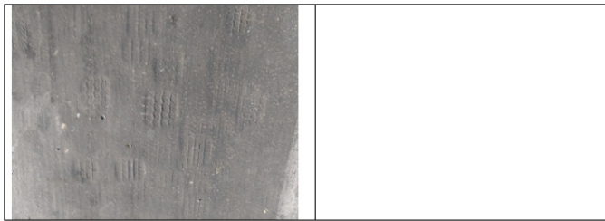
Figure 8 Traces of tire dents on the road surface after vehicles were left static for a few dozen minutes while queuing to take the ferry, Ajim side (photo R. Ben Slama, the ferry, Djerba, Tunisia, July 2023).
