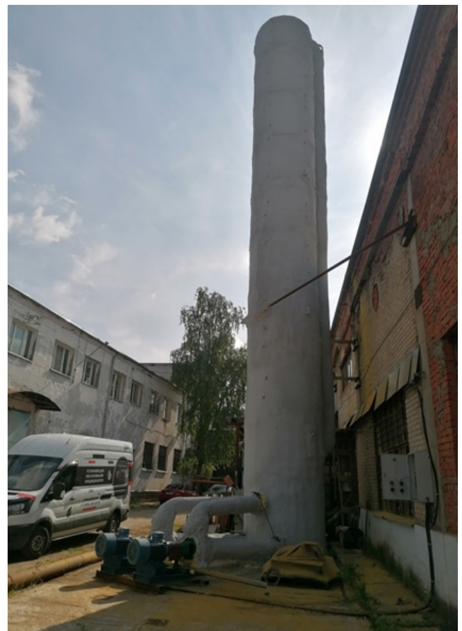
Figure 1 Thermal power plant, Mytishchi town, Moscow region, Russia (2024). Electrical power consumption is 50 kW, thermal power output is 60 kW.
