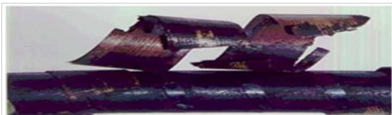
Figure 5 Exposed Copper Screens.
