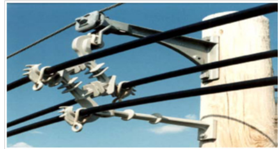
Figure 3 Typical Mounting of Triple Sheathed Spacer Cable.
