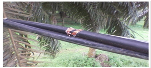
Figure 8 Damaged Outer Sheath by Squirrel Bite.
