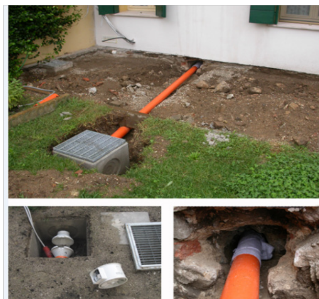
Figure 5 Remediation technique via outer suction point: a PVC pipe coated with non-woven fabric is driven into the ground under the building and then channelled to a fan located in external concrete cube.
