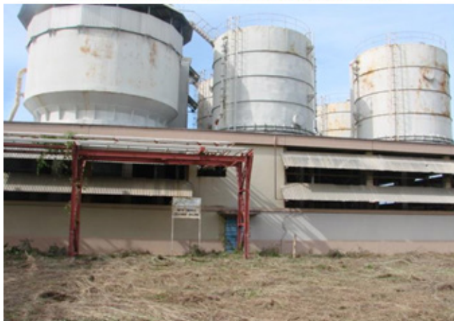
Figure 4 Production of demineralized water for boilers & turbines.
