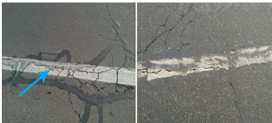
Figure 5 Cracking and sealing at asphalt surface.
