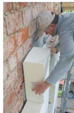
Figure 5 Exterior wall with separation of the load-bearing layer and the thermal insulation layer (two-layer wall). In hot climates, the insulating layer is very advantageously placed on the interior side, in cold climates on the exterior side of the home. 5
