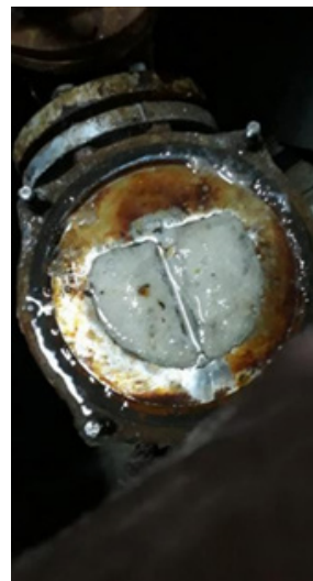
Figure 5 Mucilage effects on Seawater Inlet filters. 17
