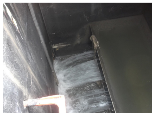
Figure 3 Unloader in operation without automatic monitoring.
