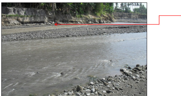
Figure 7 Riverbank collapse at the conjunction between Pabelan-Progo River.
