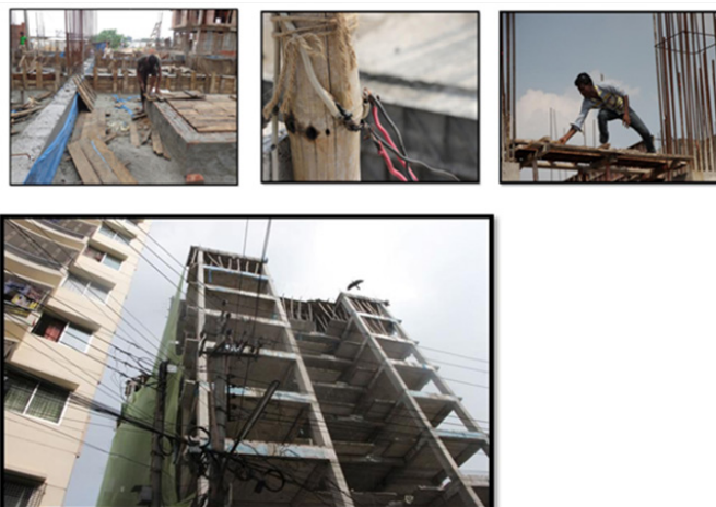
Figure 1 Some pictures safety and hazard scenario.
