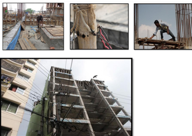
Figure 1 Some pictures safety and hazard scenario.
