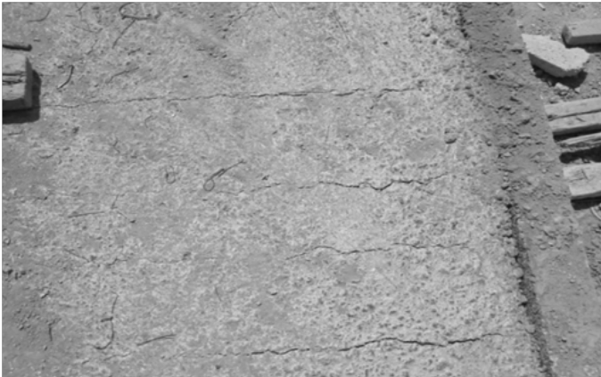
Figure 9 Cracking of a slab.
