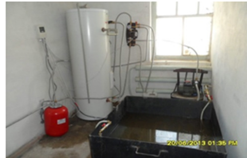
Figure 3 Heliosystem of heat treatment with intermediate coolant (boiler, electronic controller, pump). Pilot plant.
