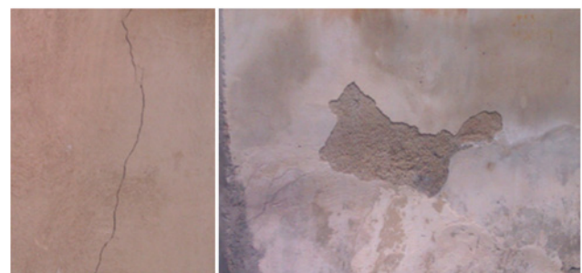
Figure 5 Issues in investigated buildings fracture poor material quality.
