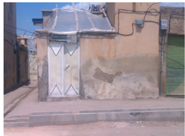
Figure 4 Vulnerable building with irregularities through the height of the buildings.
