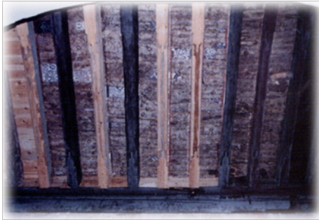
Figure 2 An image clarifies the deterioration and depletion of the tramps in the northern west shrine of El-Dashtoshy mosque, Port Said Street, Cairo.
