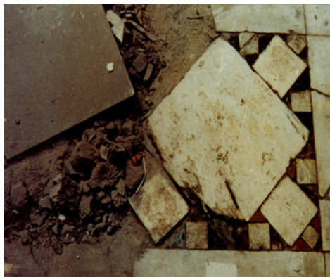
Figure 4 Architectural conservation works-deterioration of scrap marble for some flooring units, El- Kekhya mosque, Opera square, Cairo before conservation.
