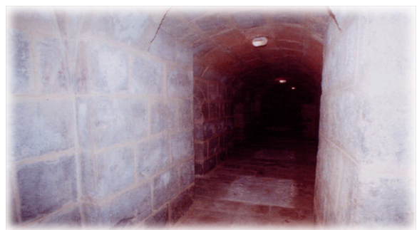
Figure 12 Ground water elevation in basement corridor in El-Dashtoodhy Mosque-Port Said After maintenance.
