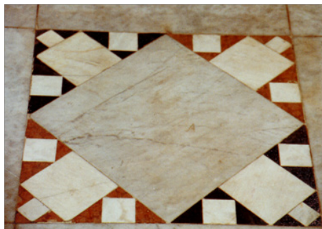
Figure 5 Architectural conservation works-deterioration of scrap marble for some flooring units, El-Kekhya mosque, Opera square, Cairo (after conservation).
