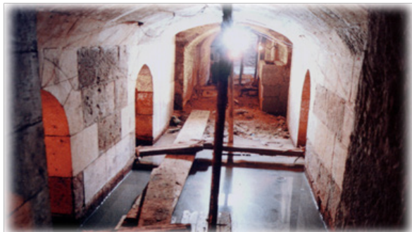
Figure 11 Ground water elevation in basement corridor in El-Dashtoodhy Mosque-Port Said.
