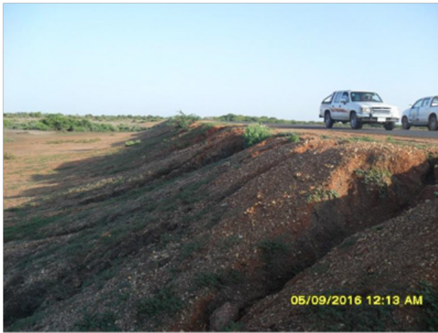
Figure 7 Picture shows the eroded side slopes of National Road.
