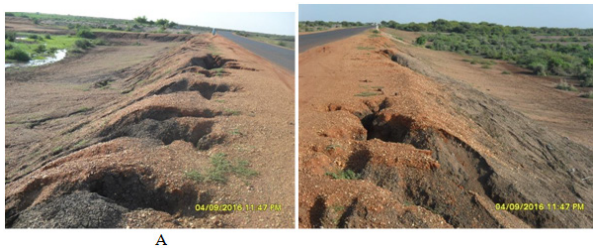
Figure 8 Pictures show the degree of eroded slope along National road.
