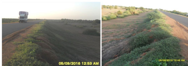
Figure 12 Existing natural local grass and (Mesquite) plant covered part of National Road side slope.
