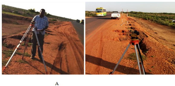
Figure 9 Surveying & Engineering measures Studies showing the eroded section of the Road.
