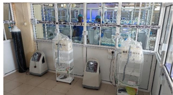
Figure 1 UATH, respiratory support substation.
