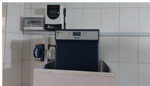
Figure 4 Solar sub-power station at all centres.
