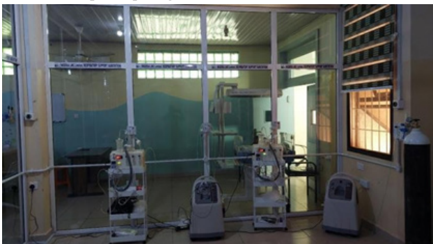
Figure 1 AKTH, Kano respiratory support substation.
