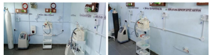
Figure 1 Two NDUTH Yenagwa Substations (left – outborn, right – inborn sections).
