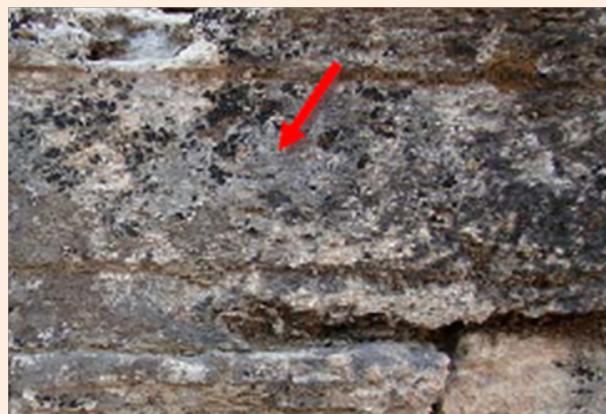
Figure 3: Thick and hard fungal stains.
