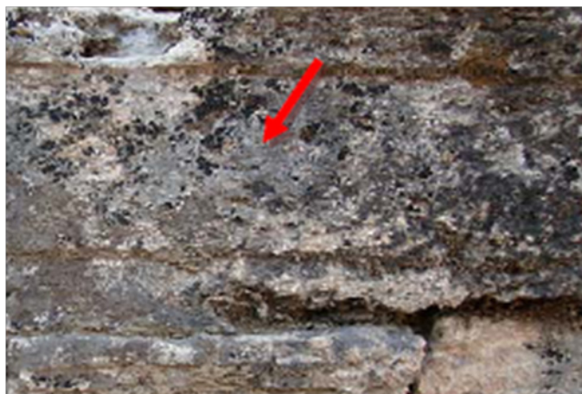
Figure 3 Thick and hard fungal stains.
