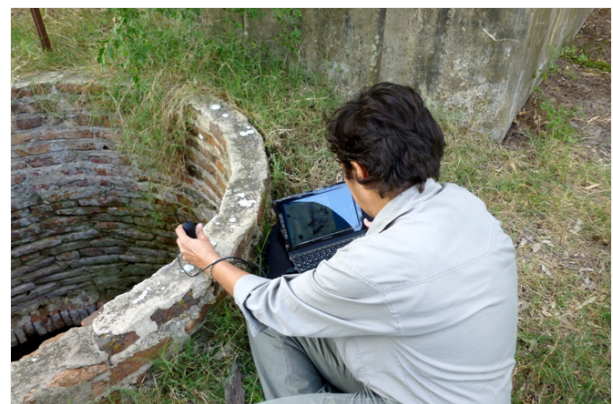
Figure 4 Dr. Mariel A López recording by USB microscopy the deterioration of the bricks of the edge of large water well located at the archaeological site SV2.
