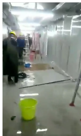
Figure 1B Example #2 still image frame from a video post of water leak.
