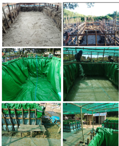
Figure 2 Pond design and construction. (A) Pond digging. (B) Framing of the pond. (C) Setting up the blower pipe. (D) water filling into the pond. (E) Terracing with pond. (F) cabin and store with ponds.
