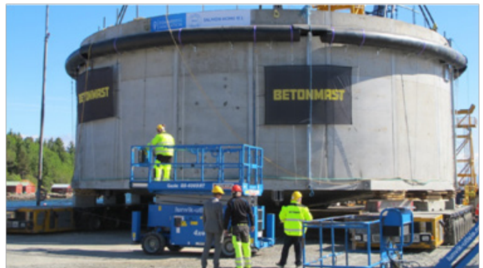
Figure 2 Olav Olsen Tank(photo courtesy of Tor Ole Olsen).
