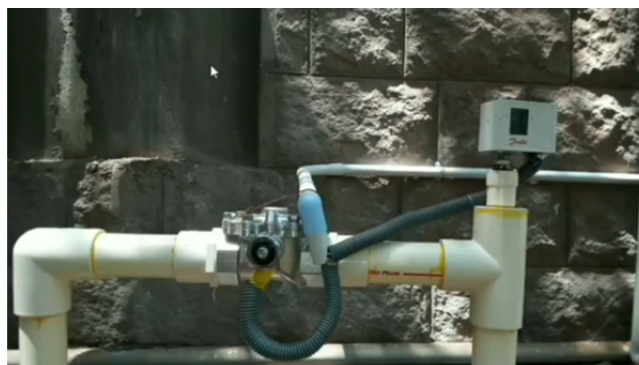
Figure 5 Automatic value control for overhead tank.
