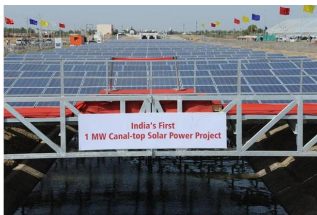
Figure 1 Canal solar Panel. 5
