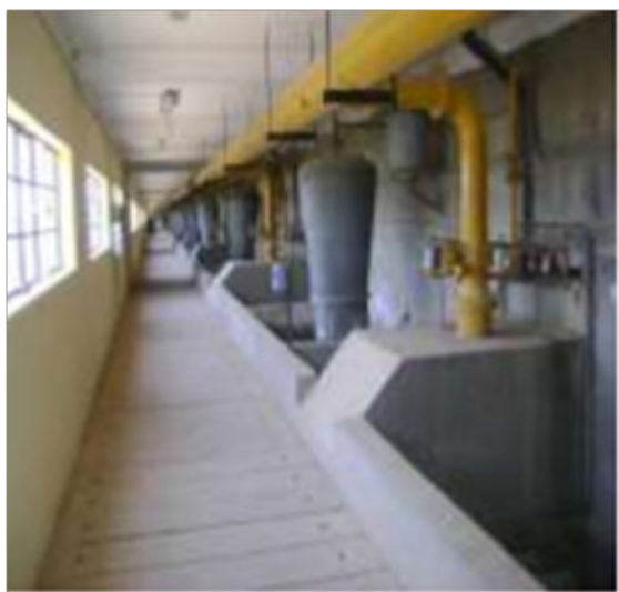
Figure 7 Filters galleries of the KNWTP.
