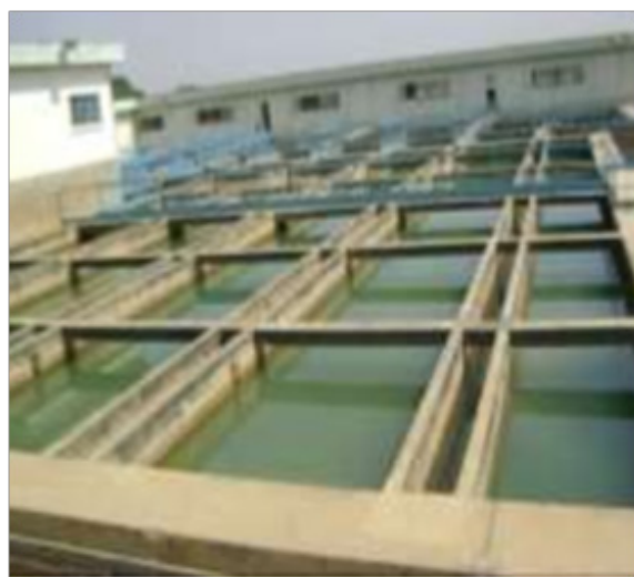
Figure 6 Sedimentation basin KNWTP.
