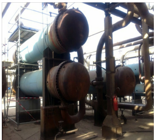
Figure 1 Picture of the E101 CBA heat exchanger.
