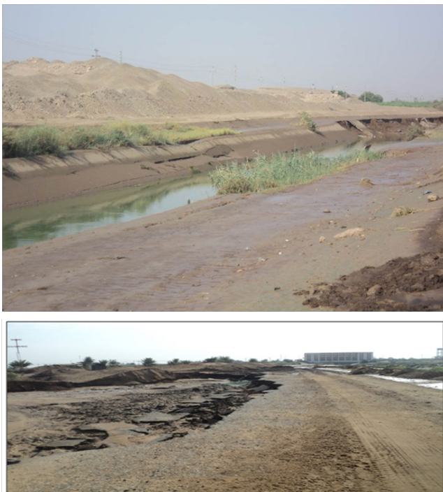
Figure 2 The extent of waste water flooding to the irrigation channel in Kom Ombo. Note the dimensions of the concrete-lined channel and the damages to some areas in the cross-section (top) and the impact of this induced flash flood on a nearby road (bottom).
