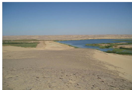
Figure 7 Formation of the new waste water lake in Al Ballanah after repairing and supporting the earth-fill dam.
