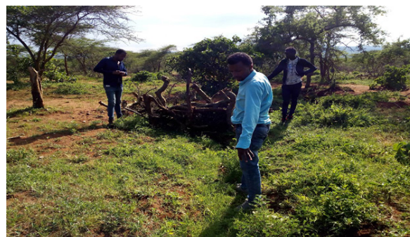
Figure 5 Change of ground cover due to sieve structure installed in the gully.
