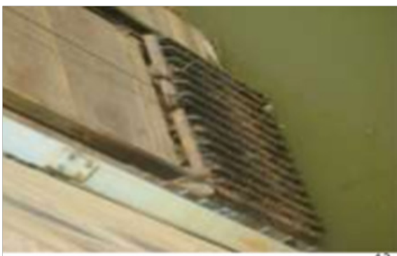
Figure 3 Screen bars of the intake section.
